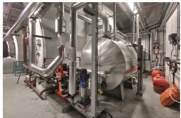
A part of City Hall’s thermal centre, linked to a monitoring system. ©Paris City Hall
