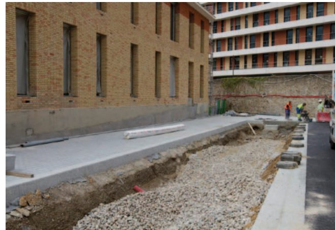
Ditch in the making at Broussais Hospital (14 th ) © Mairie de Paris, DVD
