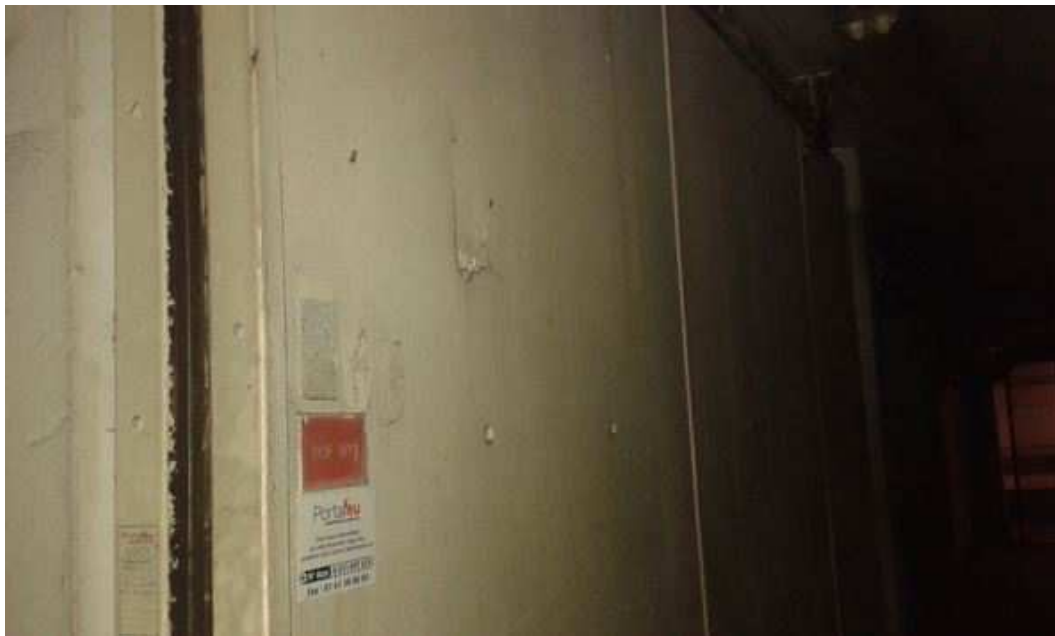
Station service 1 - Porte coupe feu - Plaque fibre ciment
