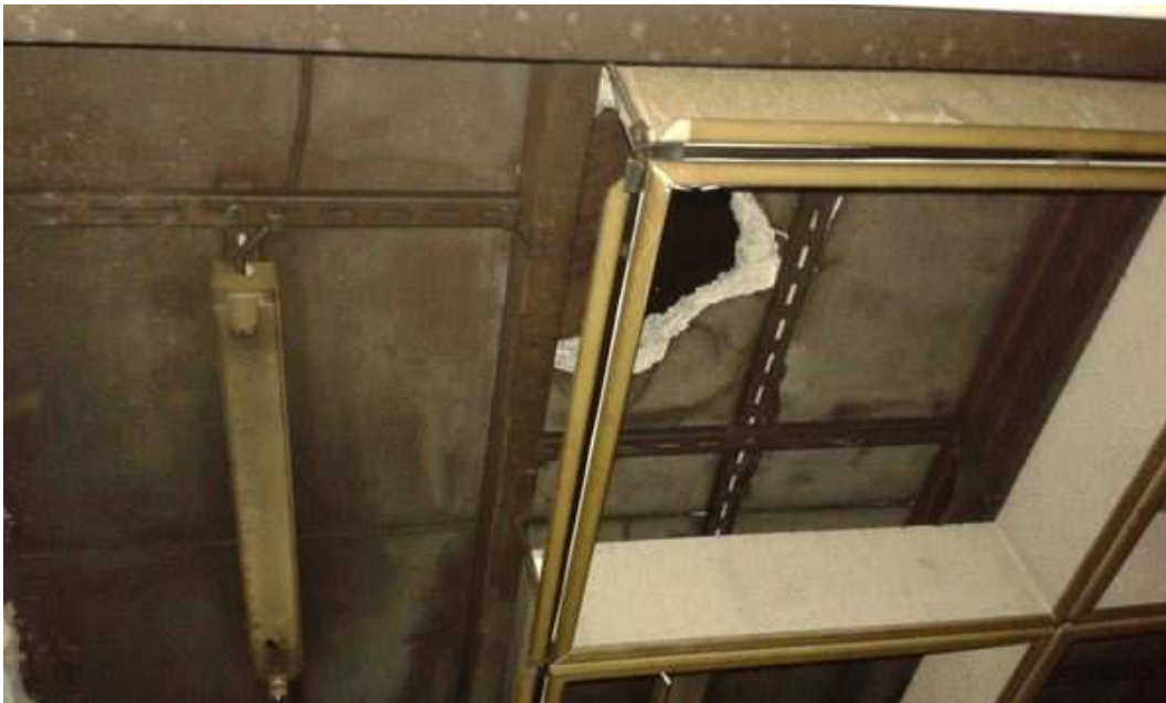
Station service 2 - Plafond - Plaque fibre ciment
