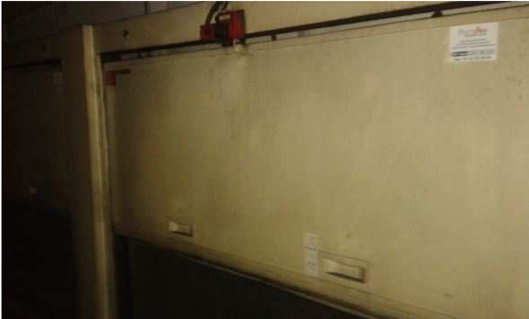
Station service 2 - Clapet coupe feu - Plaque fibre ciment
