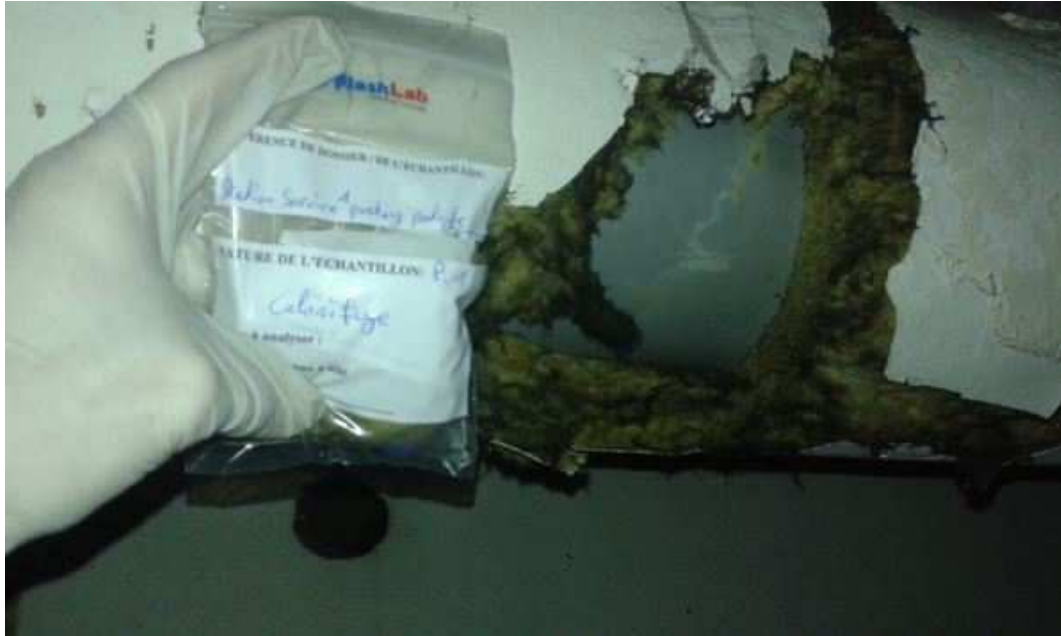
P1 - Station service 1 - Conduit - Calorifugeage
