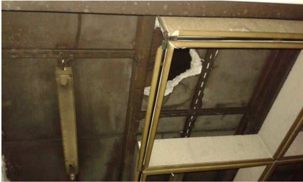
Station service 2 - Plafond - Plaque fibre ciment
