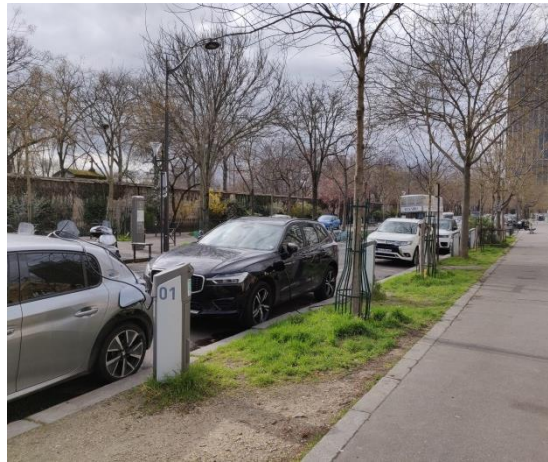
Borne de recharge – boulevard Edgar Quinet
