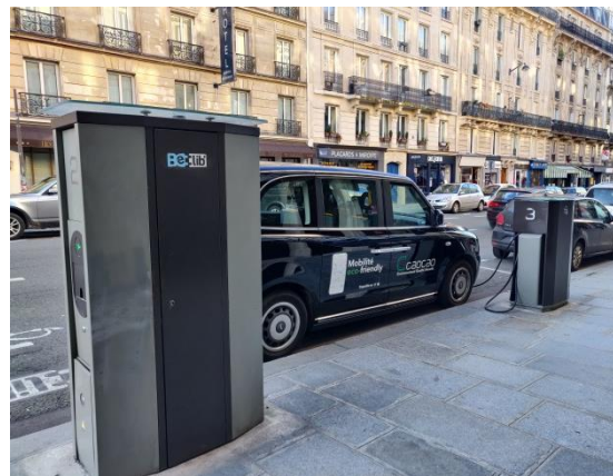
Station de recharge Belib – rue Monge
