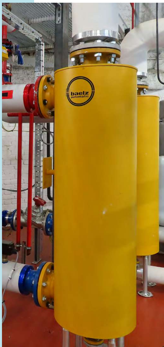
Boiler room, 8 th district town hall @Cyril Abbas
