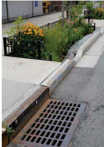
Right-of-way Bioswale, Brooklyn
